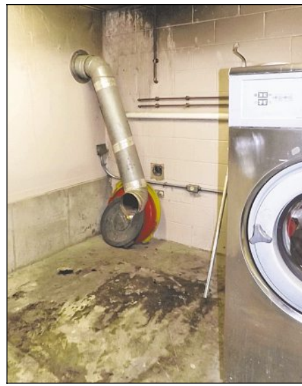
A New Year's Eve Fire destroyed the Boone County Animal Shelter's industrial dryer and caused smoke damage. PROVIDED
